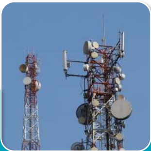
ANTENNA BASE STATION
