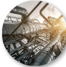
AIR-CONDITIONING SYSTEM (HVAC)
